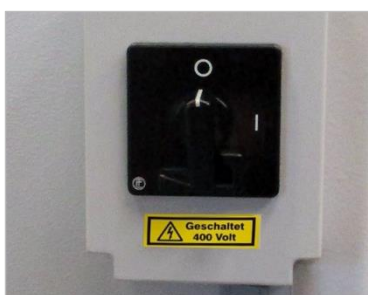
Figure 5: Lockable main switch
